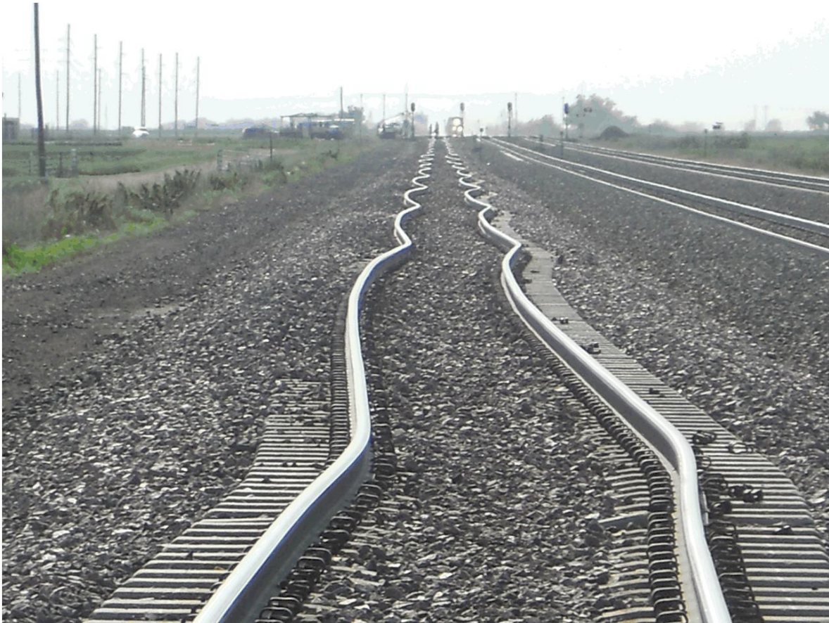
Figure 2 A heat damaged railroad track.
