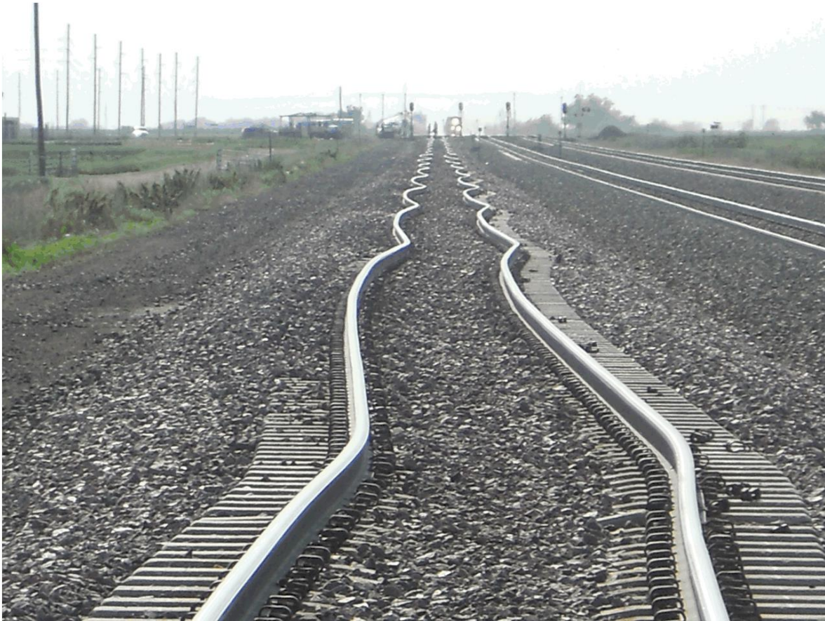
Figure 2 A heat damaged railroad track.
